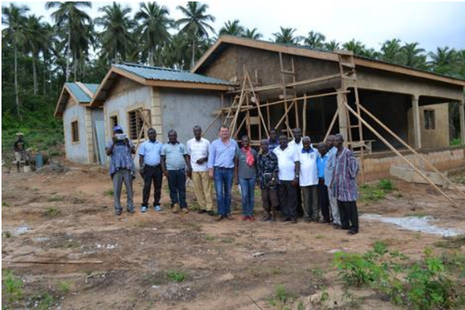
Above: the Foundation team by a clinic being constructed in Nawule in the Jomoro area of Ghana. The project will be completed by August.
