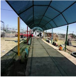
Maria Mbhele Installation of a new roof for a creche at Maria Mbhele in South Africa.
