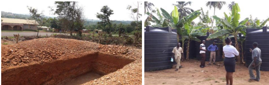
Above: (left) Foundations being dug for a 12 seater toilet at Oboadaka and (right) polytanks are donated by the community of Akraman to collect water pumped by boreholes which will be drilled by the Foundation
