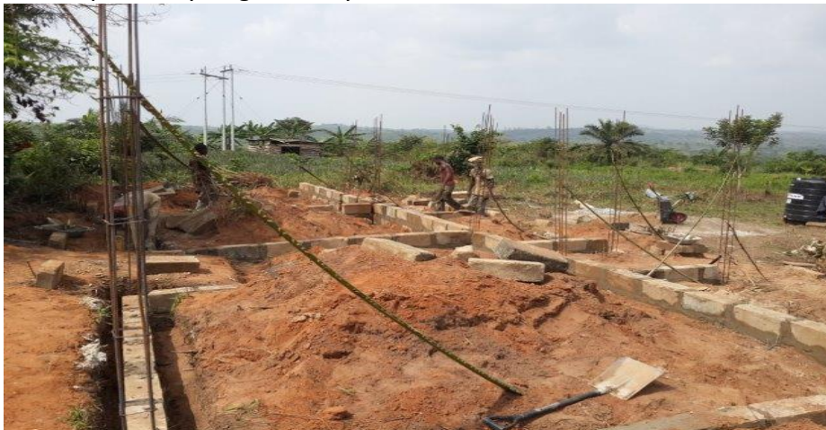
Above: work starts at Yaw Duodu to build a three bedroom teachers block
